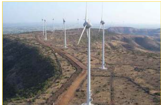
Moil's Wind turbine generator
